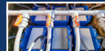
Image of Cerafiltec membranes installation for the upgrade at an existing waste-water treatment facility.
