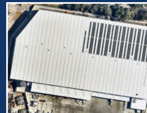
Rooftop solar panels installed at Charter Hall asset (East Logistics Park, Queensland, Australia)
